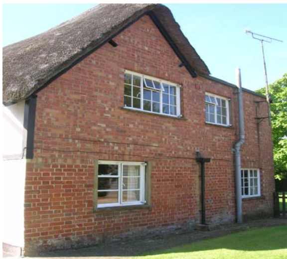
Below: An unsympathetic flat roofed extension with unsightly waste pipes, modern windows and aerial
